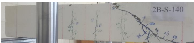
Figure 11 Cracks patterns of beam 2B-S-140
