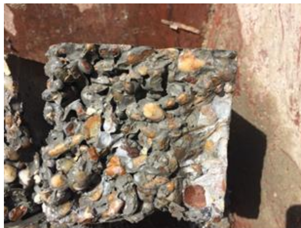
Figure 10. Photo of a cross section of prism made from a reference mix failed in flexure.
